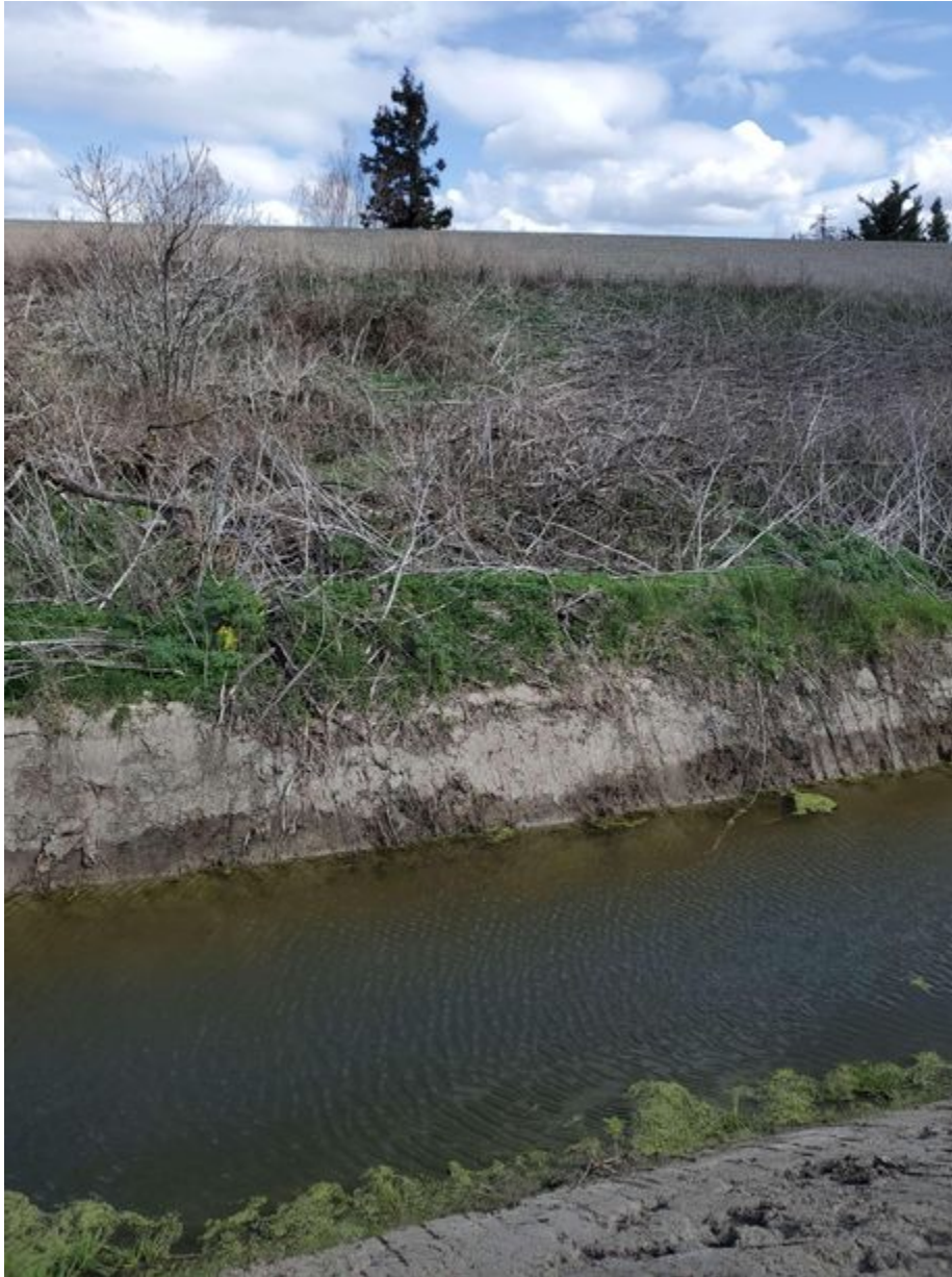
Image taken from the Ag Field, looking East. Shows the maintained bank of the ag ditch, and the levee in the background.
